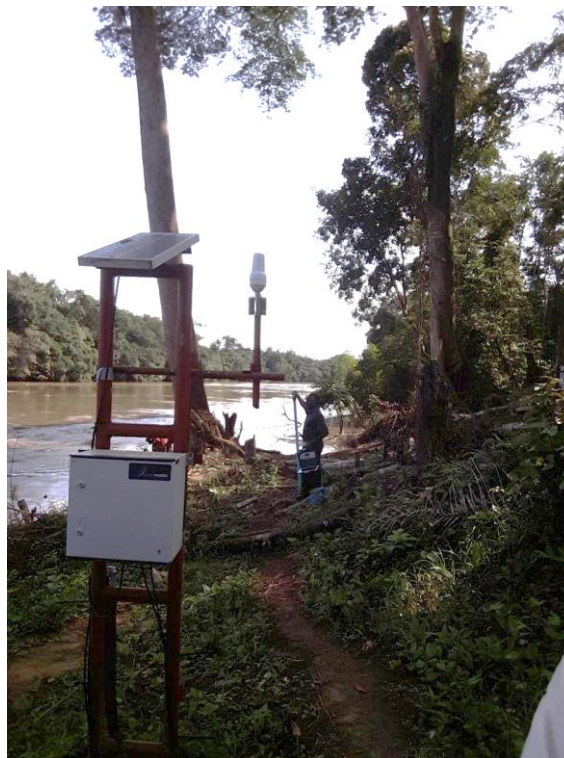
Photo 1 – Haindi gauging station cubicle. PV panel and satellite antenna. In the background, LHS staff downloading readings from one of the two pressure-cell sensor onto a portable computer.
